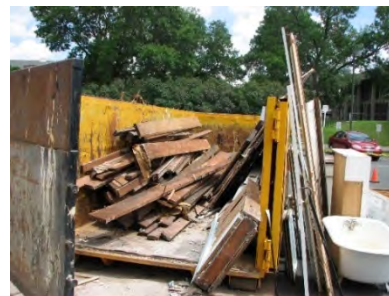
Figure 26. Deconstruction is the process of dismantling buildings in a manner that allows for materials to be reused.
