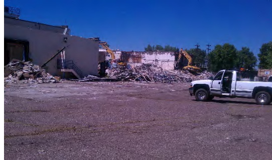
Figure M. Through careful demolition and remediation of the Twin Cities Army Ammunition Plant, 93% of removed materials were recycled or reused.
