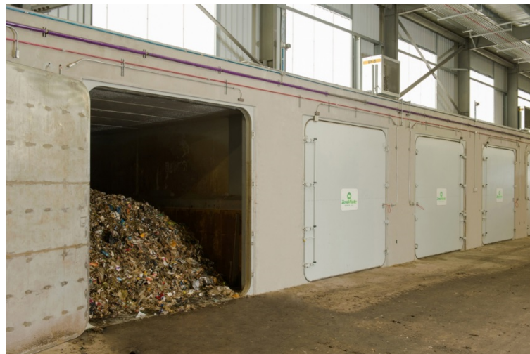
Figure 3 ZeroWaste Energy Development Company Facility, San Jose, California www.zwedc.com
